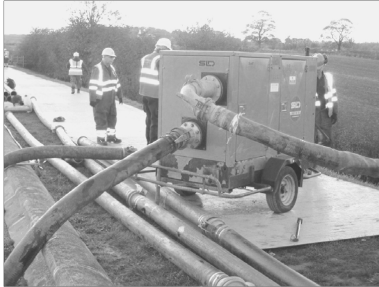
Figure 4. Suction Pump Set Up
